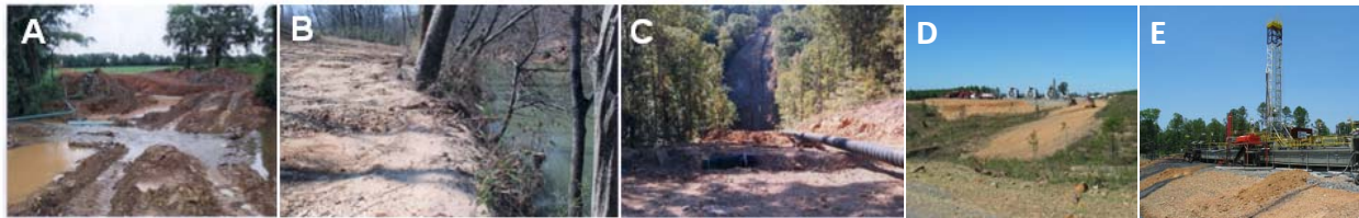
Fig. 1. Sedimentation from installation and maintenance of natural gas wells. A) Stream trenching for laying pipe under a small stream; b) ditch and fill activities along the riparian corridor of a stream; and C) slope clearing of vegetation to lay pipe for gas distribution, D) compressor sites, roads, and E) gas wells. Photos courtesy of Lindsey Lewis, USFWS
