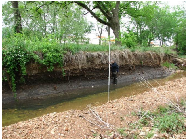
Figure 1 Accelerated streambank erosion on Turtle Creek in the Illinois River watershed.
